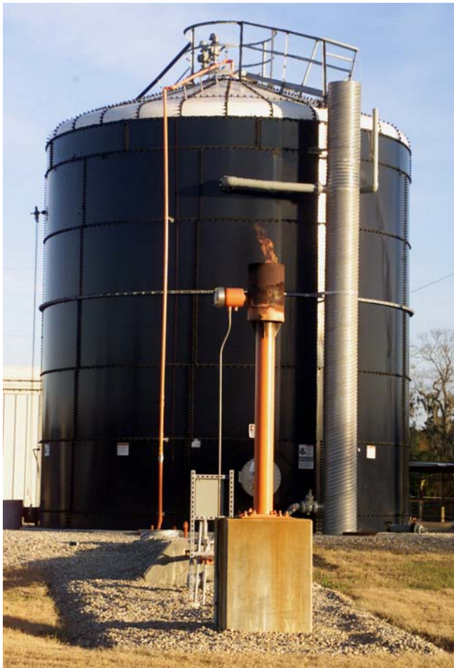
Figure 3: Fixed-Film Anaerobic Digester.
